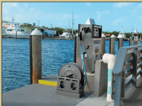
Gasoline & Diesel Fuel
